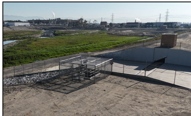
Outlet Control Gate/Rubber Dam System
